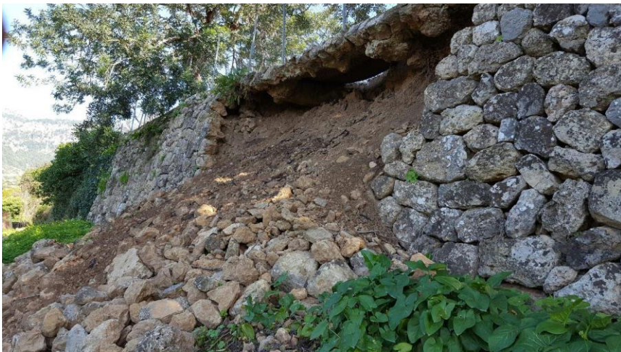
Figure 9 - Collapsed dry-stone wall as a result of a lack of maintenance. Source: Author's research.
