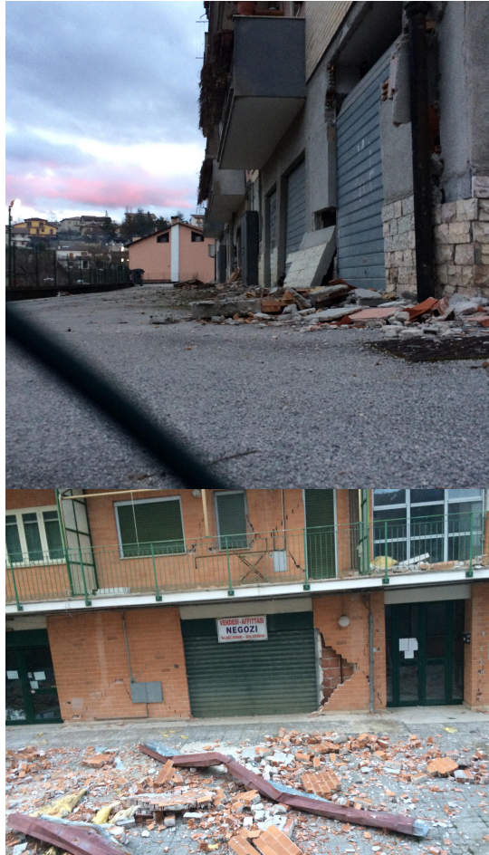
Figure 3 - Effects of earthquake on XX century city.
